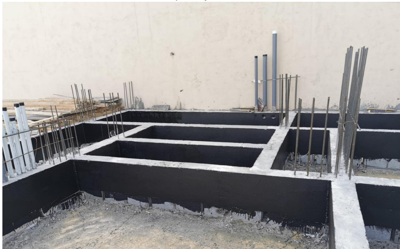
Insulation and burial works of cement grout foundation and ground slab works
