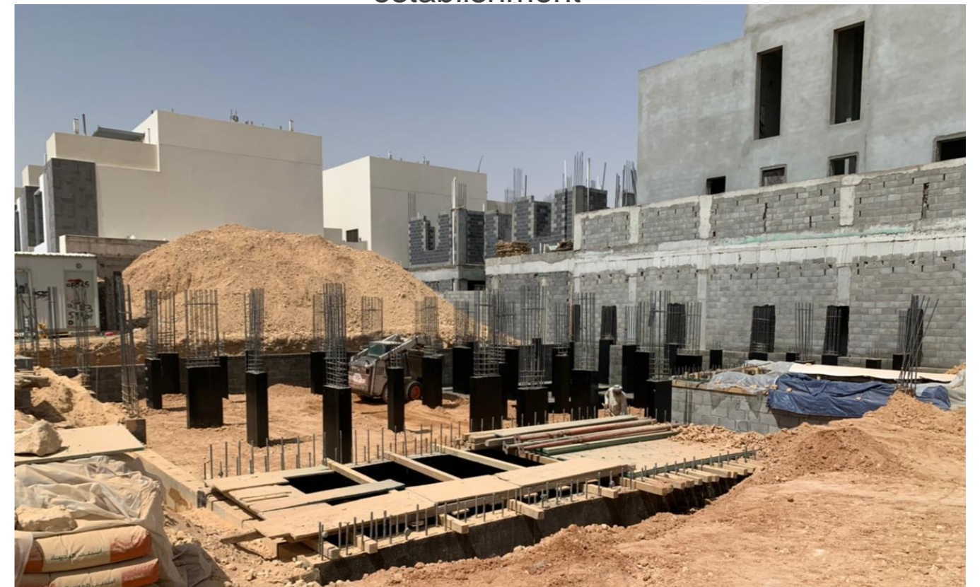
Determine the filling layers on the pad foundation, as well to the columns and start filling work
