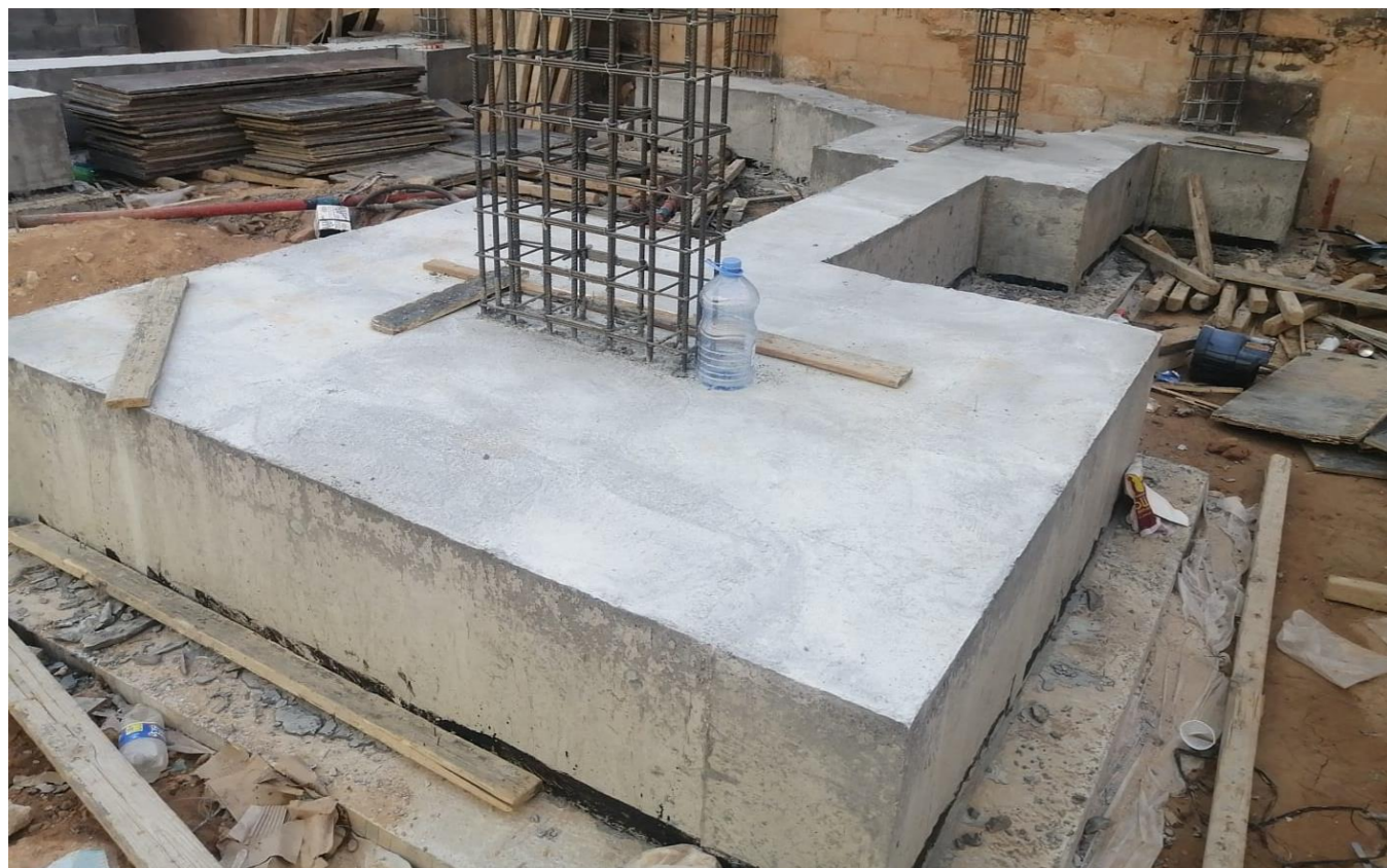
Insulation and burial works of cement grout foundation and ground slab works
